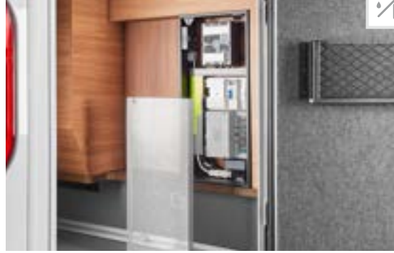
Electrical centre in scooter garage, easily accessible
