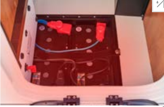
Heated battery centre with main power switch. Standard: Gel batteries 2 x 80 Ah, easily accessible, optional Lithium ion battery, 90 Ah including battery computer and separate touch display.
